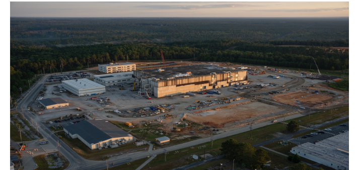
U.S. DOE Savannah River Plutonium Processing Facility // Aiken, SC
