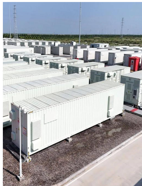
100 MW / 4h battery storage project
